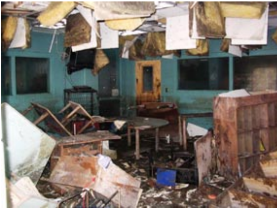
The interior of the Martin Luther King Library in New Orleans, LA was totally destroyed.
